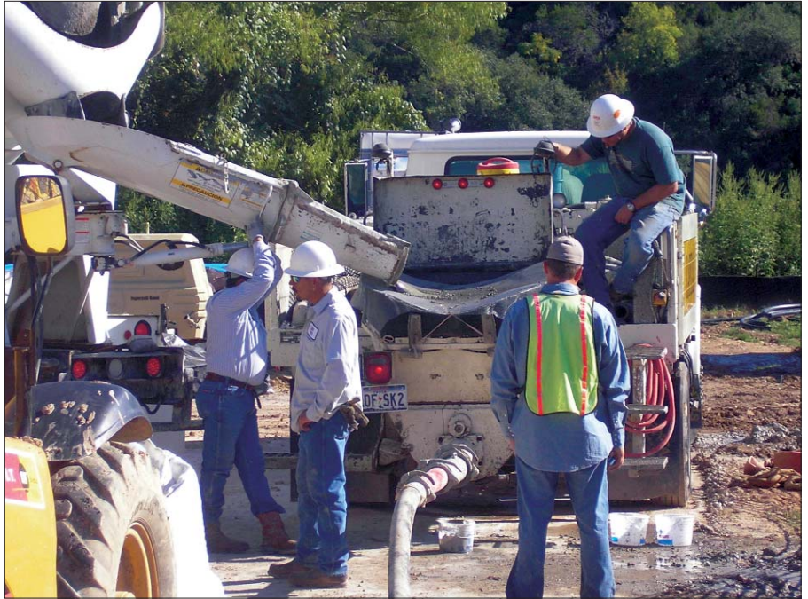
Constellation Group has performed grouting work using HDD technology, expanding the capabilities of the pipeliner to reach areas previously unavailable.
